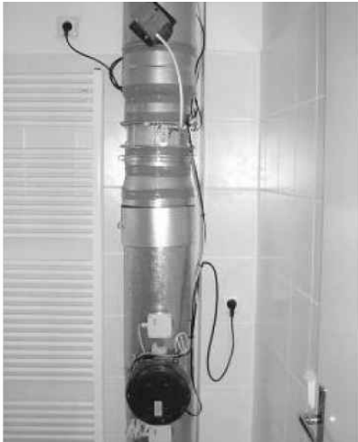
(c) Exhaust Chimney
